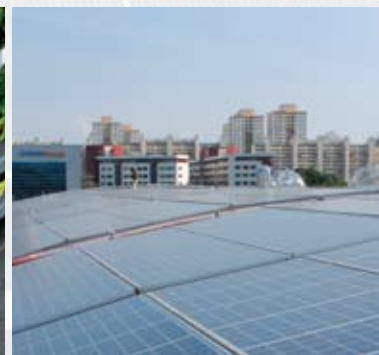
PV installation in Singapore
